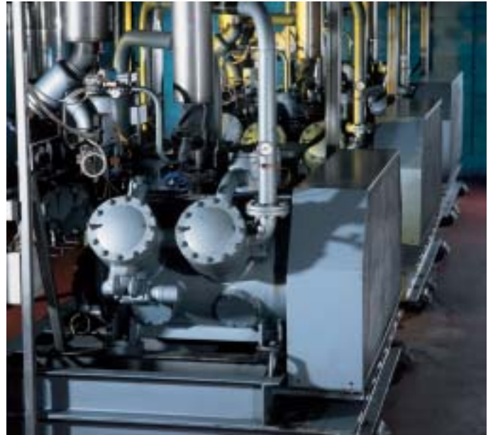
Refrigeration systems are essential for food processing and storage. This refrigeration plant includes three Grasso reciprocating compressor packages.
